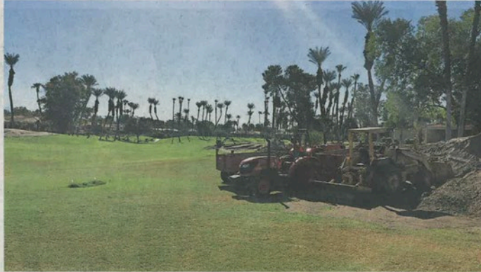
Work on the second fairway at Desert Horizons Country Club in Indian Wells includes building new bunkers.
